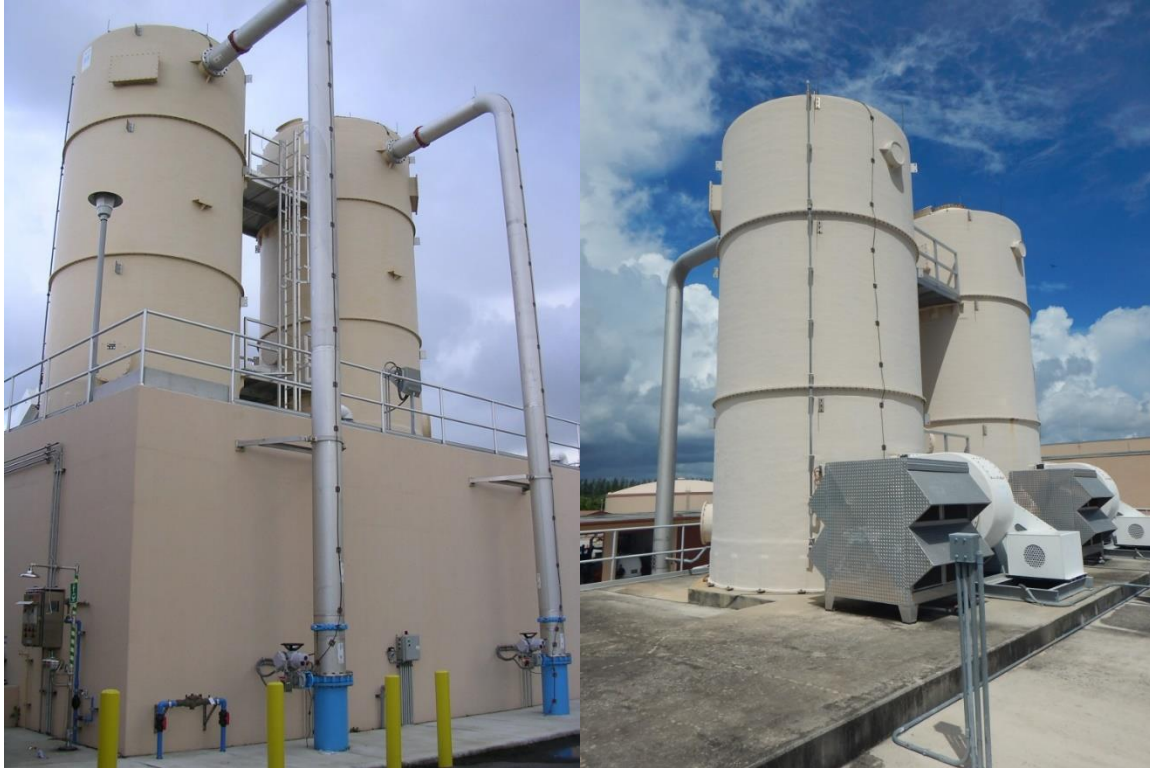
City of Hallandale Beach Water Treatment Plant Membrane Degasification Towers Photo
